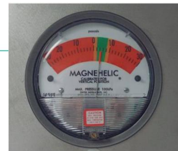
Image of room pressure gauge indicating colour-coded normal, alert & action parameters
